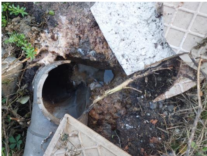
Figure 42: Absence de tampon
